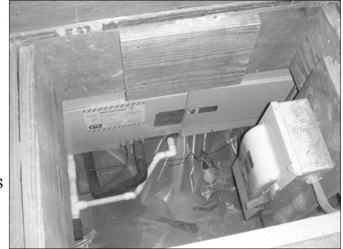
Though once more efficient than the original radiators, this unit is no longer doing its job and will be replaced.
