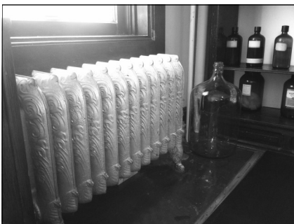
One of many radiators that provided heat for the new (1896) Pathology Department.
